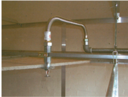
Rapidrop Sprinkler System
